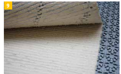
9 This results in embedding in the substrate over the entire surface. Further work takes place after the bonding of the IndorTec® THERM-E has hardened.
